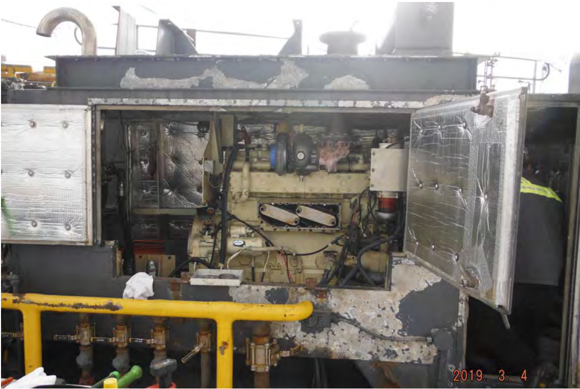
Photo No. 9 Main engine and compartment
